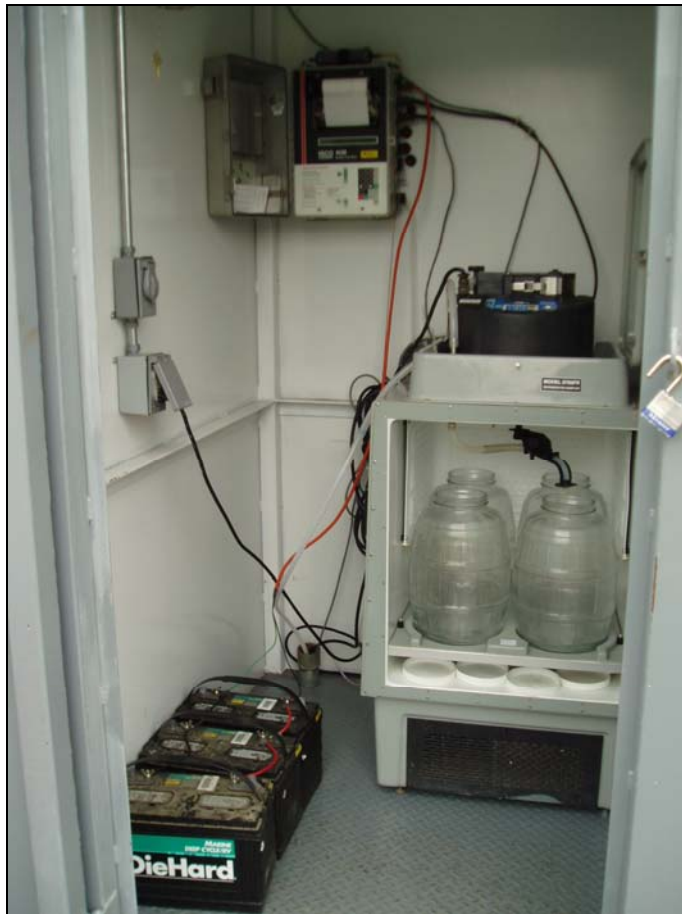
Figure 3: ISCO 6712 refrigerated sampler, ISCO 4230 flowmeter, and steel enclosure at Mass Emission site ME-VR2
