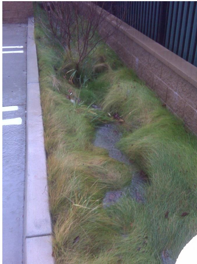
Low Impact Development infiltration BMP
