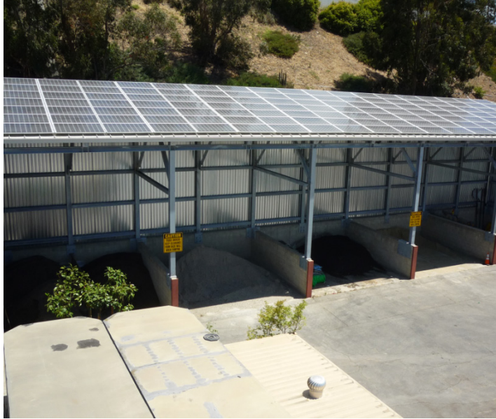
Material storage covers in Camarillo also support solar panels
