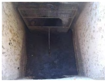
Full Capture Device Cleanout
