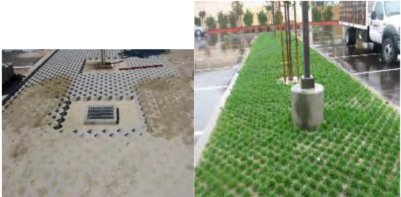
Before and after pictures of infiltration area of parking lot during construction.
