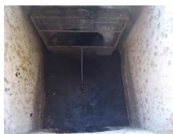
Full Capture Device Cleanout
