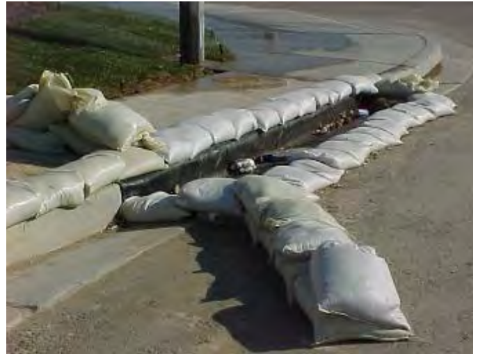
Catch basin protection
