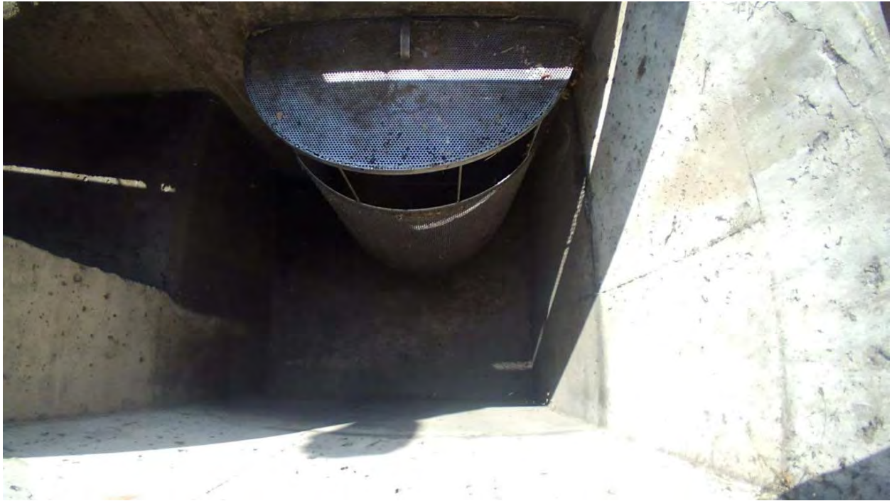
Figure 3. Full capture device after cleaning in June, 2018
