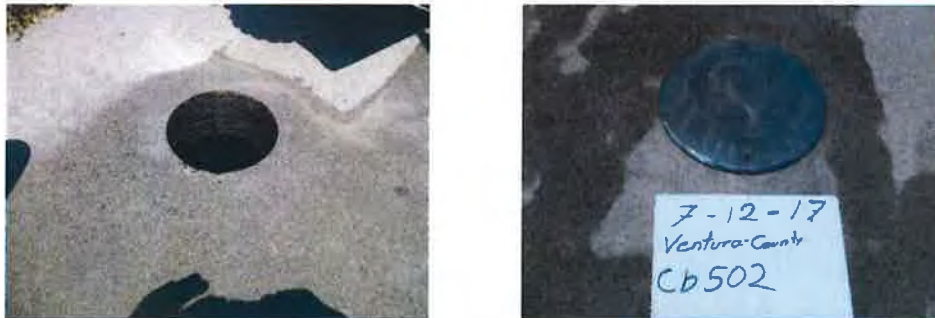
Figure 2 - Maintenance Access Port & Lid
