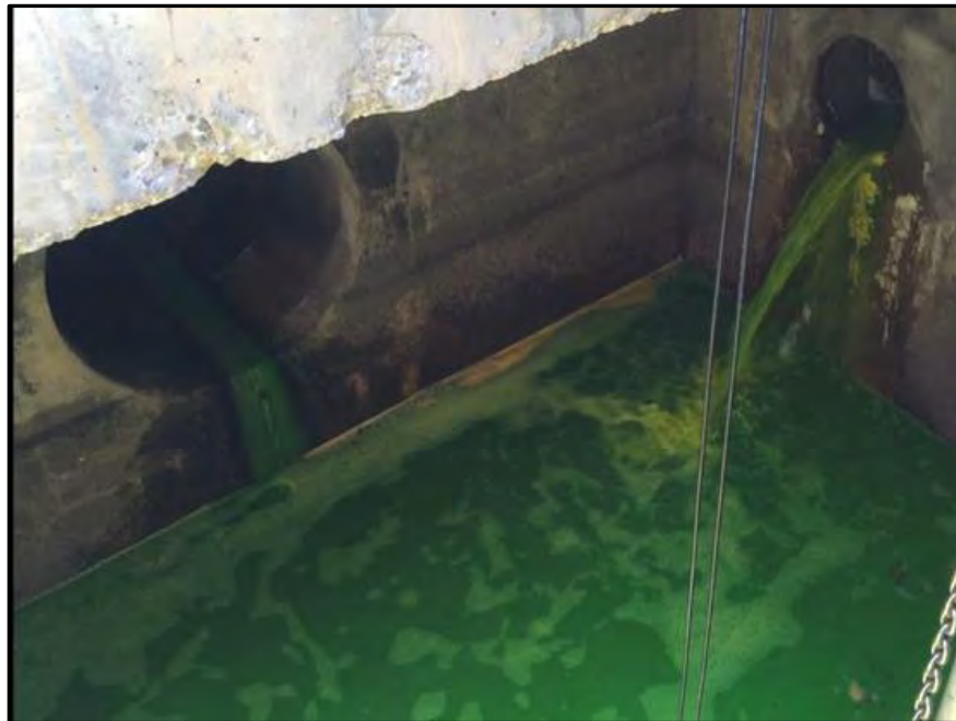
36'' and 18'' RCPs discharging to Pump Station Containment Vault (Provided by the County)
