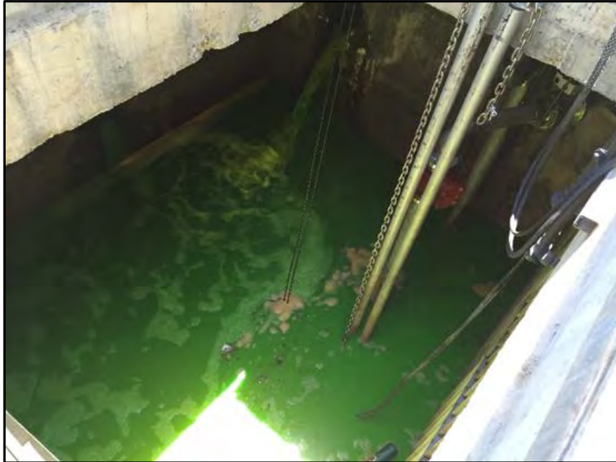
Dye Entering Pump Station Containment Vault (Provided by the County)
