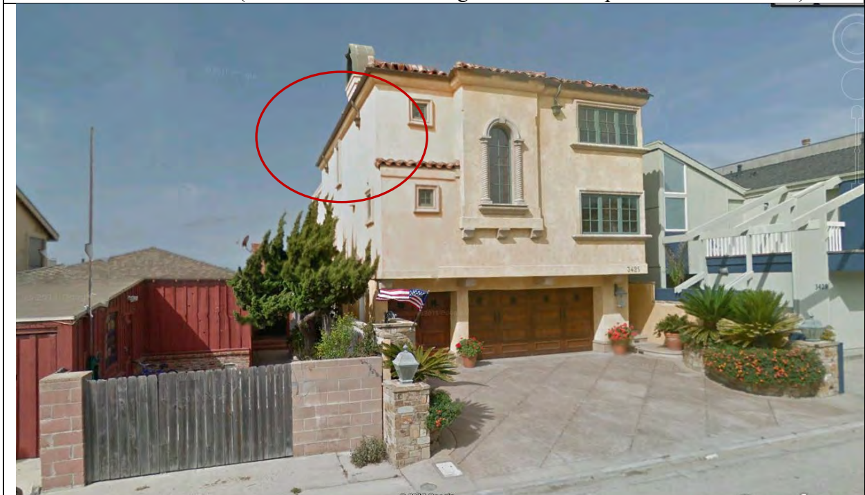
Ocean Drive 3424 – Internal routing of gutters
