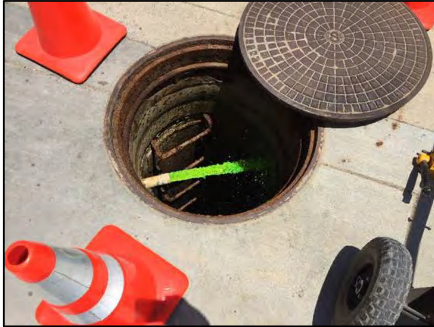
Sewer diversion pump discharging to sanitary sewer system (Provided by the County)
