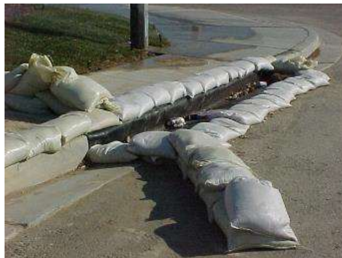
Catch basin protection
