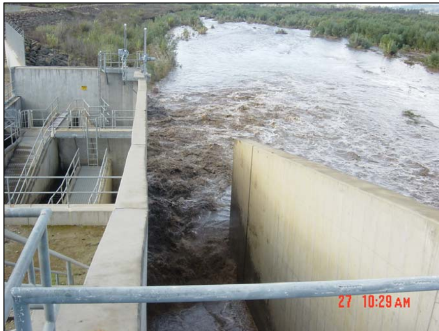
Figure 12: River Diversion Gate (Facing Downstream)
