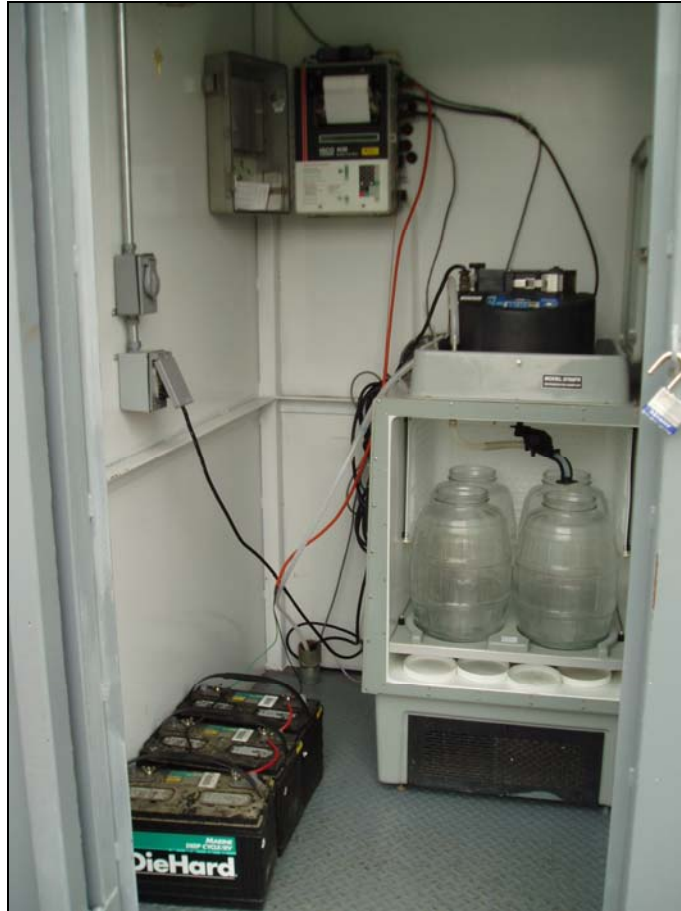
Figure 9: Newly installed ISCO 6712 refrigerated sampler, ISCO 4230 bubbler/flow meter, and steel enclosure at Mass Emission site ME-VR2 located at the Ojai Valley Sanitation District Treatment Plant
