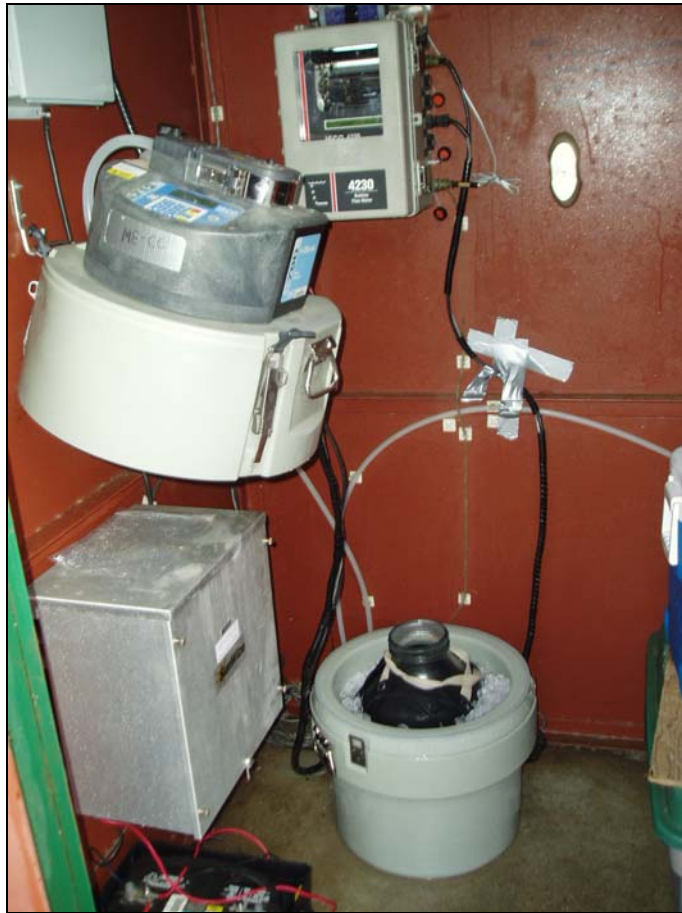
Figure 22: ISCO 6712 sampler (cover removed showing iced carboy) and ISCO 4230 bubbler/flow meter used to collect composite samples at Mass Emission site ME-CC
